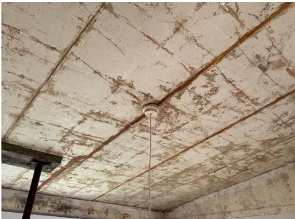
Figure 6: Typical RAAC panels condition observed during surveys
